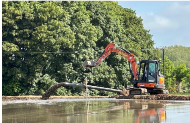
Sludge being pumped from Raynham Hall Lake into one of the lagoons
