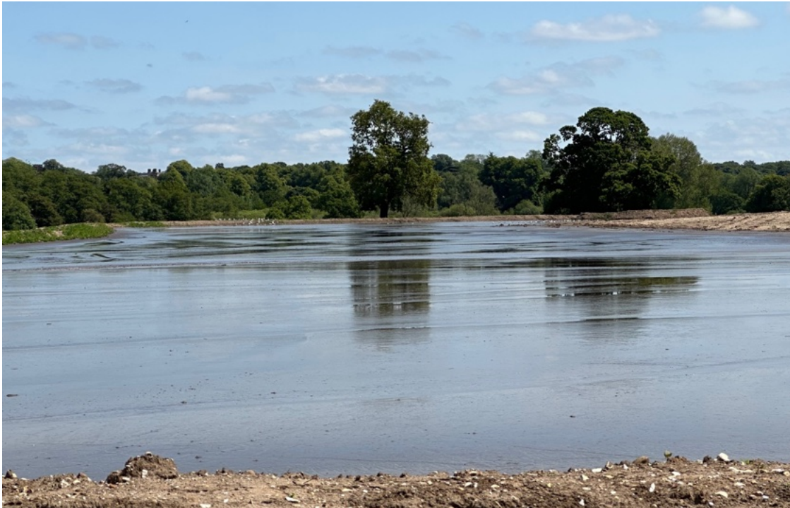
One of the temporary silt lagoons viewed from the diverted public footpath.
